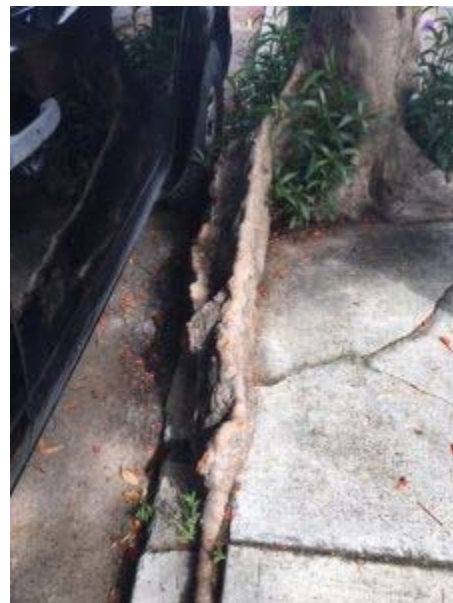
Figure 4. Damaged tree roots
