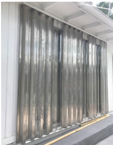
Metal/polycarbonate storm panels
